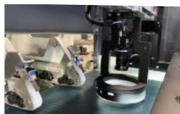
In-line inspection station
